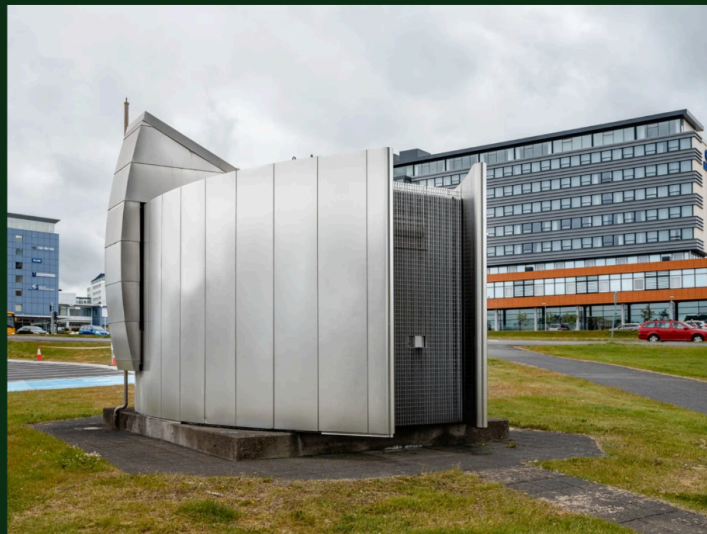
One of Veitur Utilities' low-temperature wells in City of Reykjavík.
