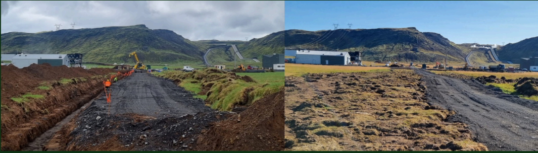
Surface restoration with local vegetation at the trench site of a water pipeline in ON Power's Geothermal Park in the summer of 2023.
