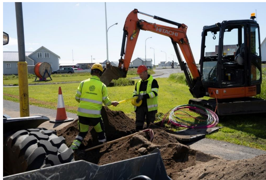
Figure 5: Retractable pipe laid in Ljósleidari trench in Stokkseyri. Photo: Arna Rut Hjartardóttir.
